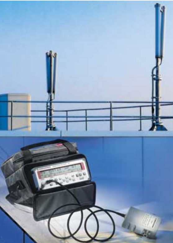
NRT is also ideal for mobile use, eg for measurements on GSM antennas
